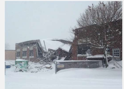
Figure 5 A collapsed building from intense wind and snowfall.
